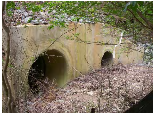
RCPs with Different Sizes and Inverts at Weaver Dairy Road Extension
