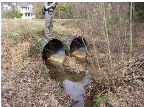
Double CMPs Projecting from Fill at Dixie Lane
