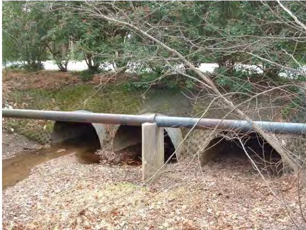
Triple CMP Arch Pipes with Sedimentation at Tinkerbell Road
