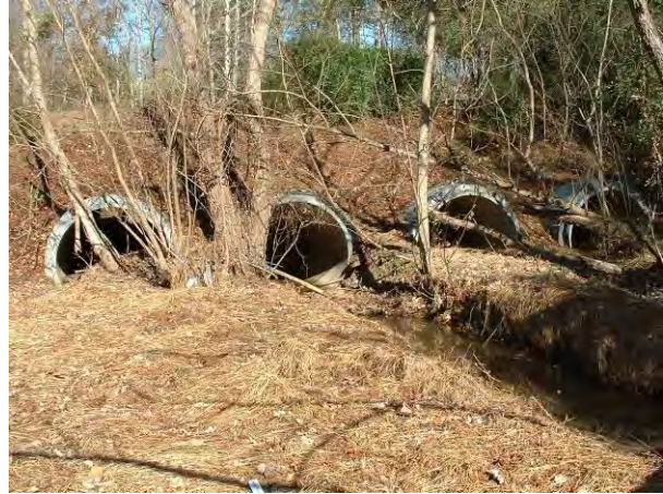
Four RCP Pipes with Excessive Sedimentation at Boxwood Drive
