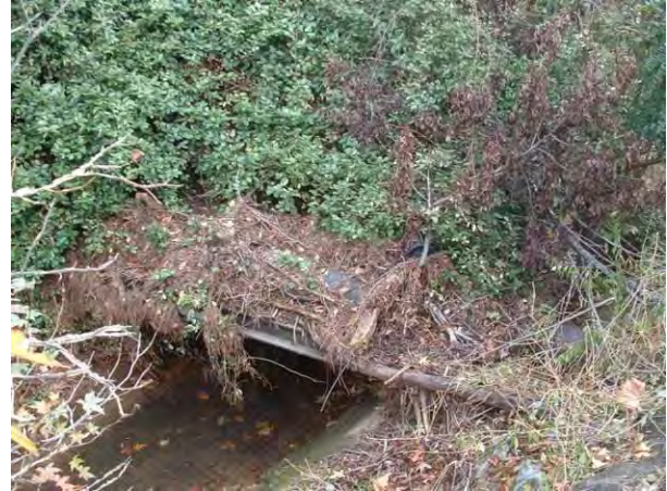
Heavy Vegetation on a Sewer Aerial & Beam
