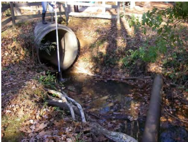
Exposed Sewer Pipe Downstream of Culvert
