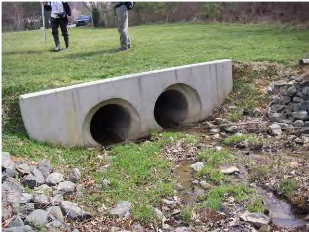
RCP Pipes with Tapered Invert at Northfield Drive
