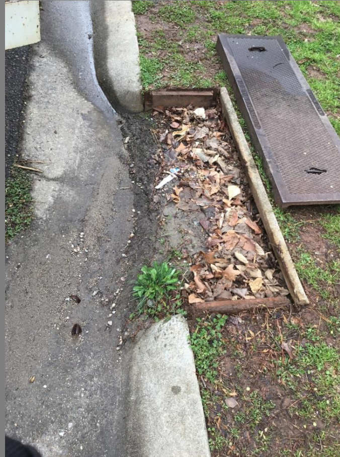
Catch basin filled with debris
