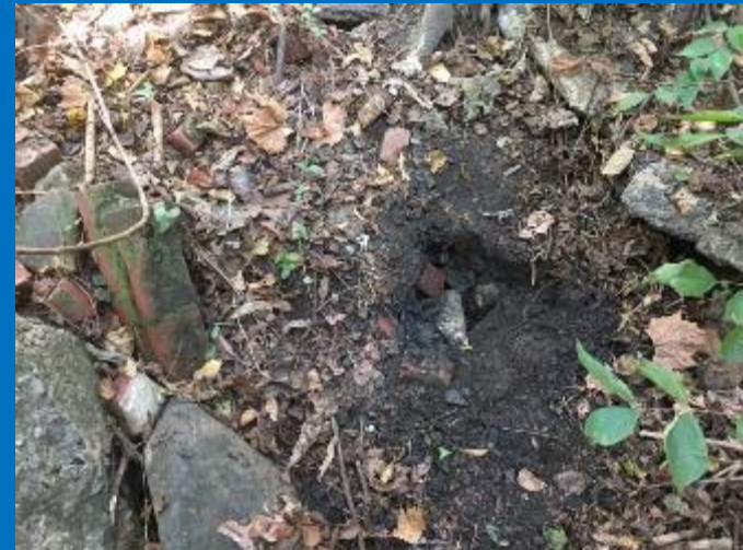
CCP Exposed At Surface
